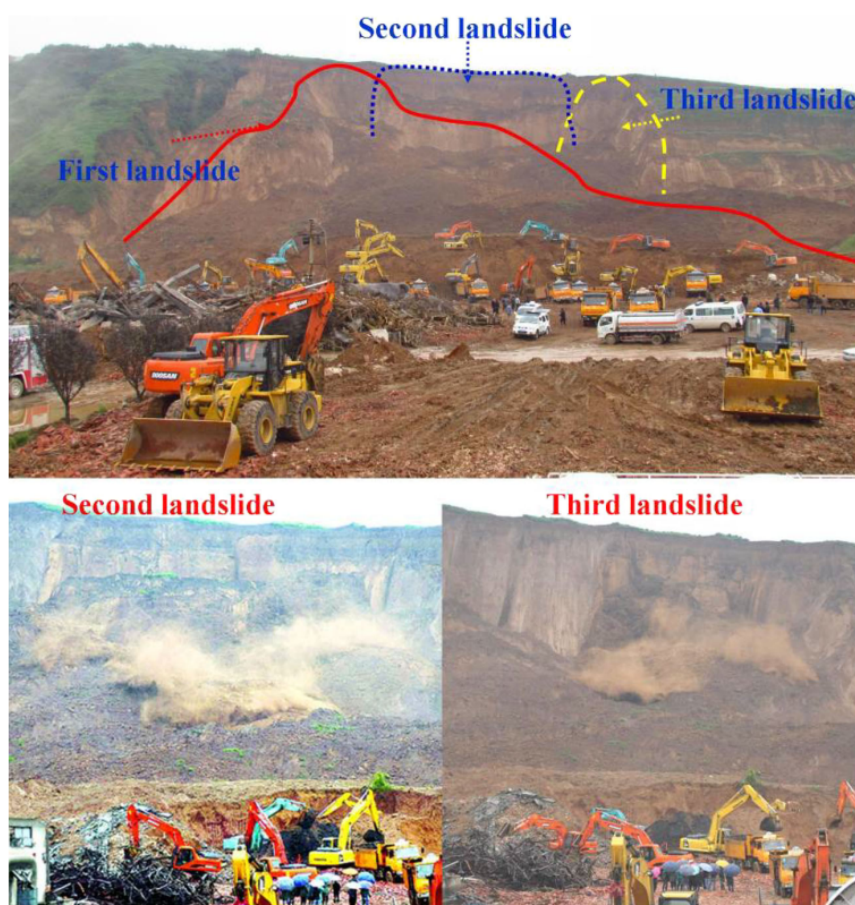
Figure 7.1: Photographs of the Baqiao landslides in September 2011.
